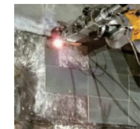
Anti-cavitation coating on hydro power station
